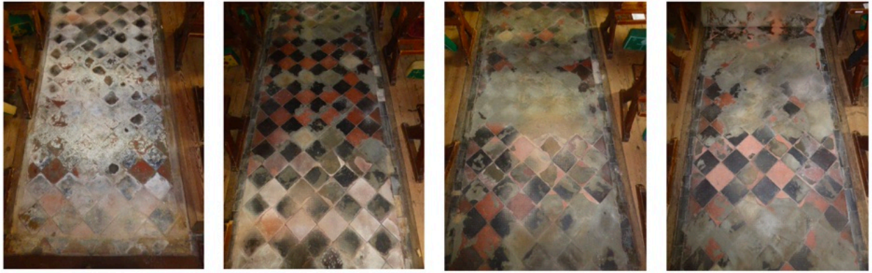
Figure 3: Taken from the Floor Investigation report 2017
